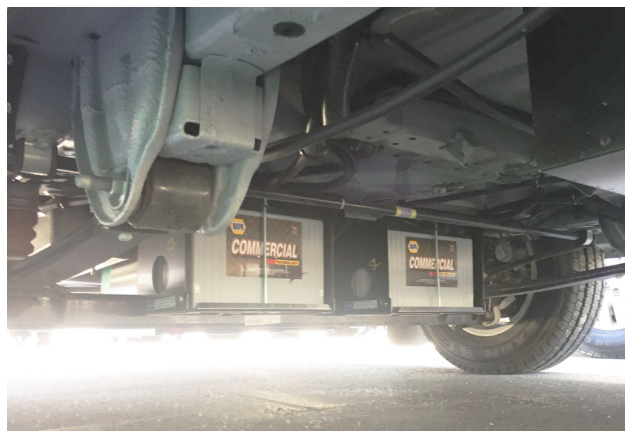
House Battery Access (Located behind rear tires)
