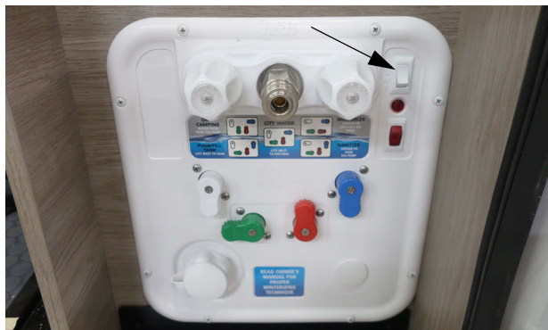
Pump switch -Typical View
